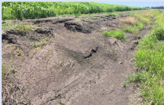
Drainage bank damage
